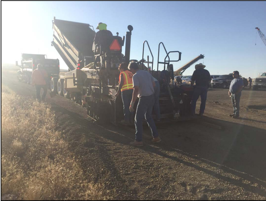
It was all hands on deck to making improvements to the roads at the training center this summer.
