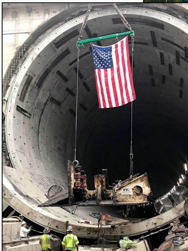
Light at the end of the tunnel. North Portal after the last Bertha piece was removed
