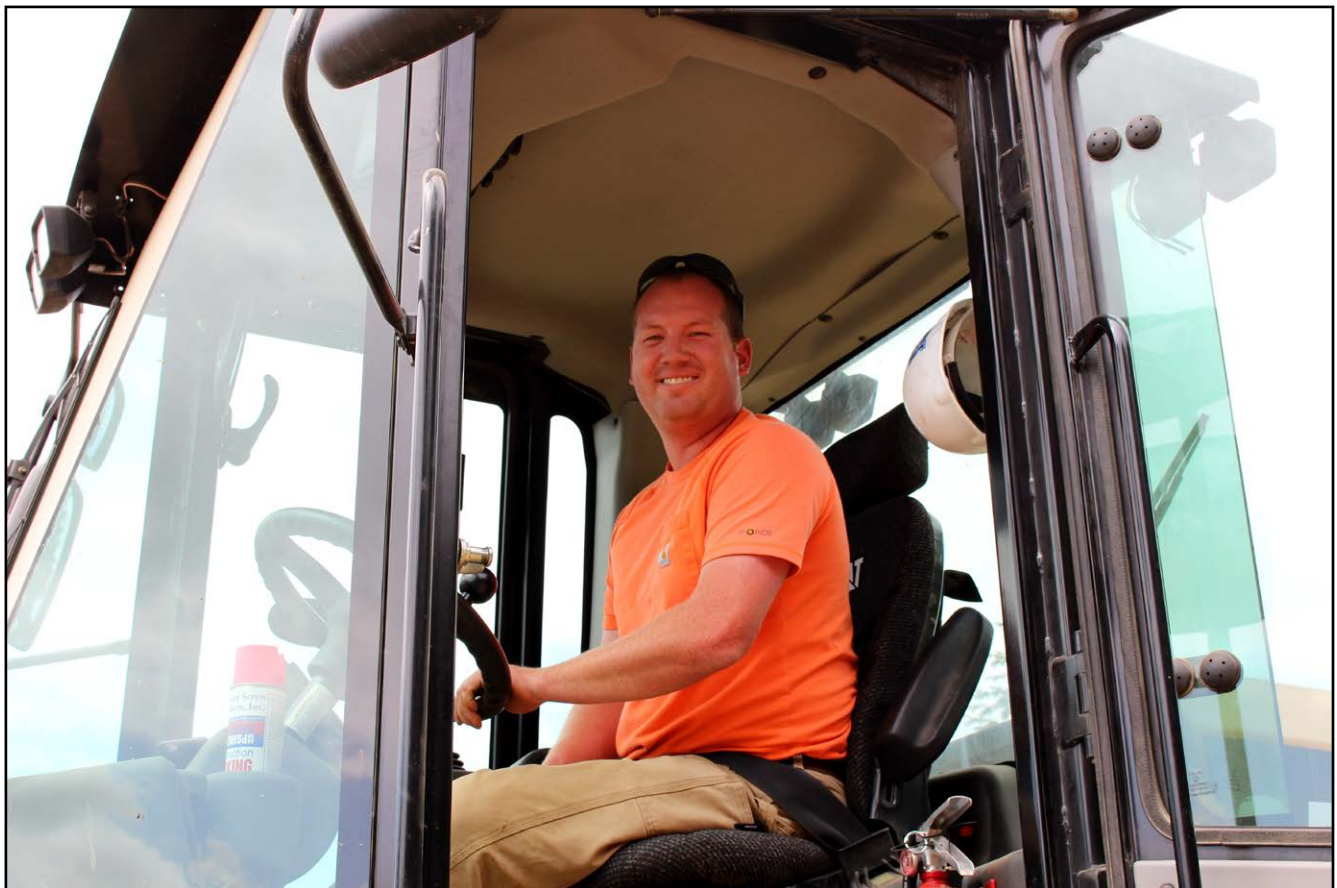
Apprentice James Gaines working hard for ICI making sure the grade is well compacted!
