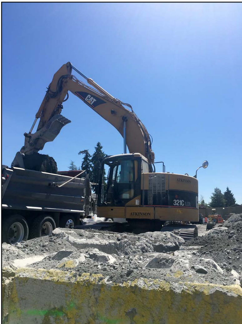
Apprentice Steve Lucas doing a great job loading trucks at the Atkinson East Link project in Bellevue.
