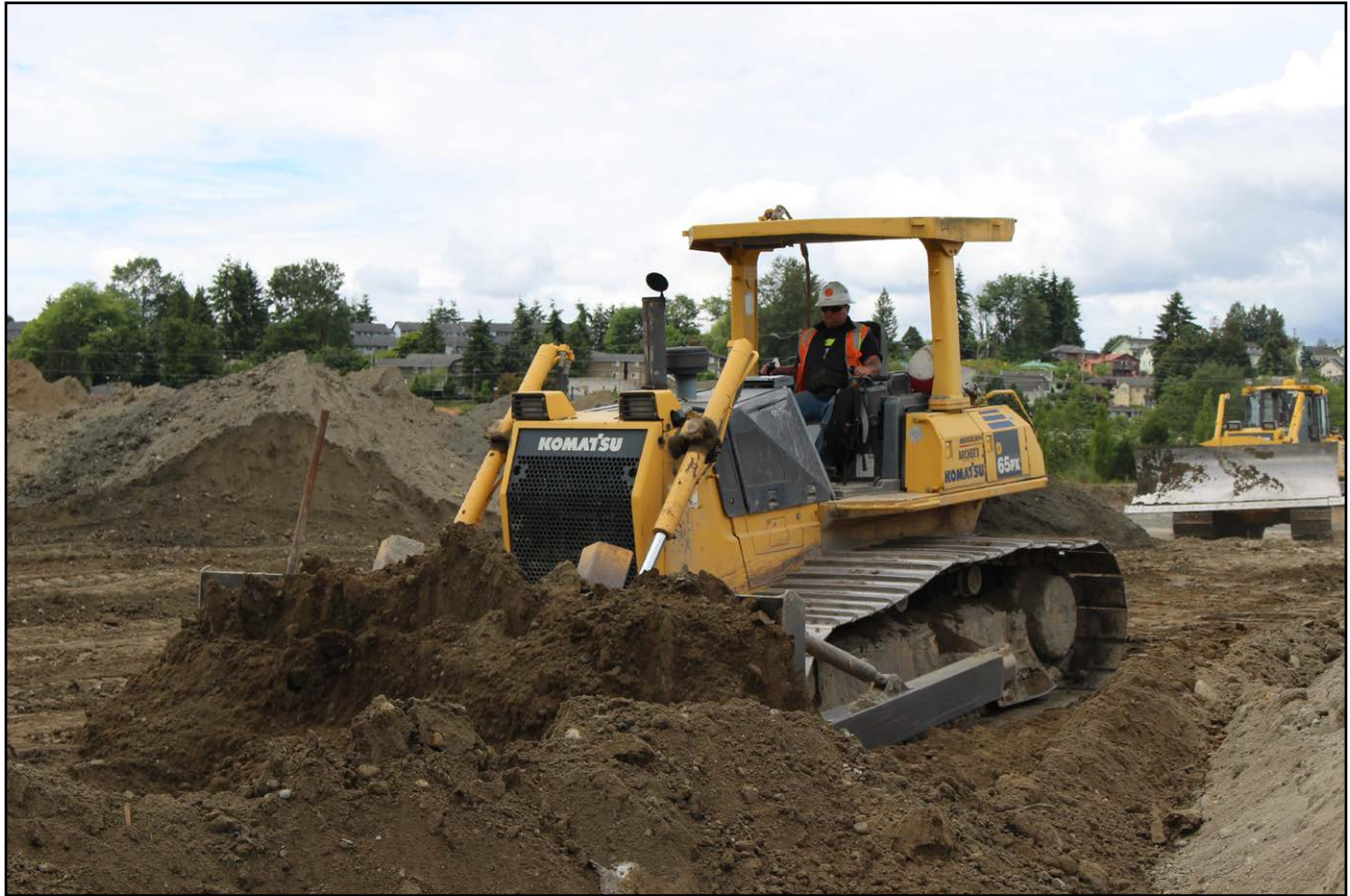
Apprentice Jaye Kessler-Walls working the fill for Archer Construction at one of the two new Fed-ex sites in Everett.
