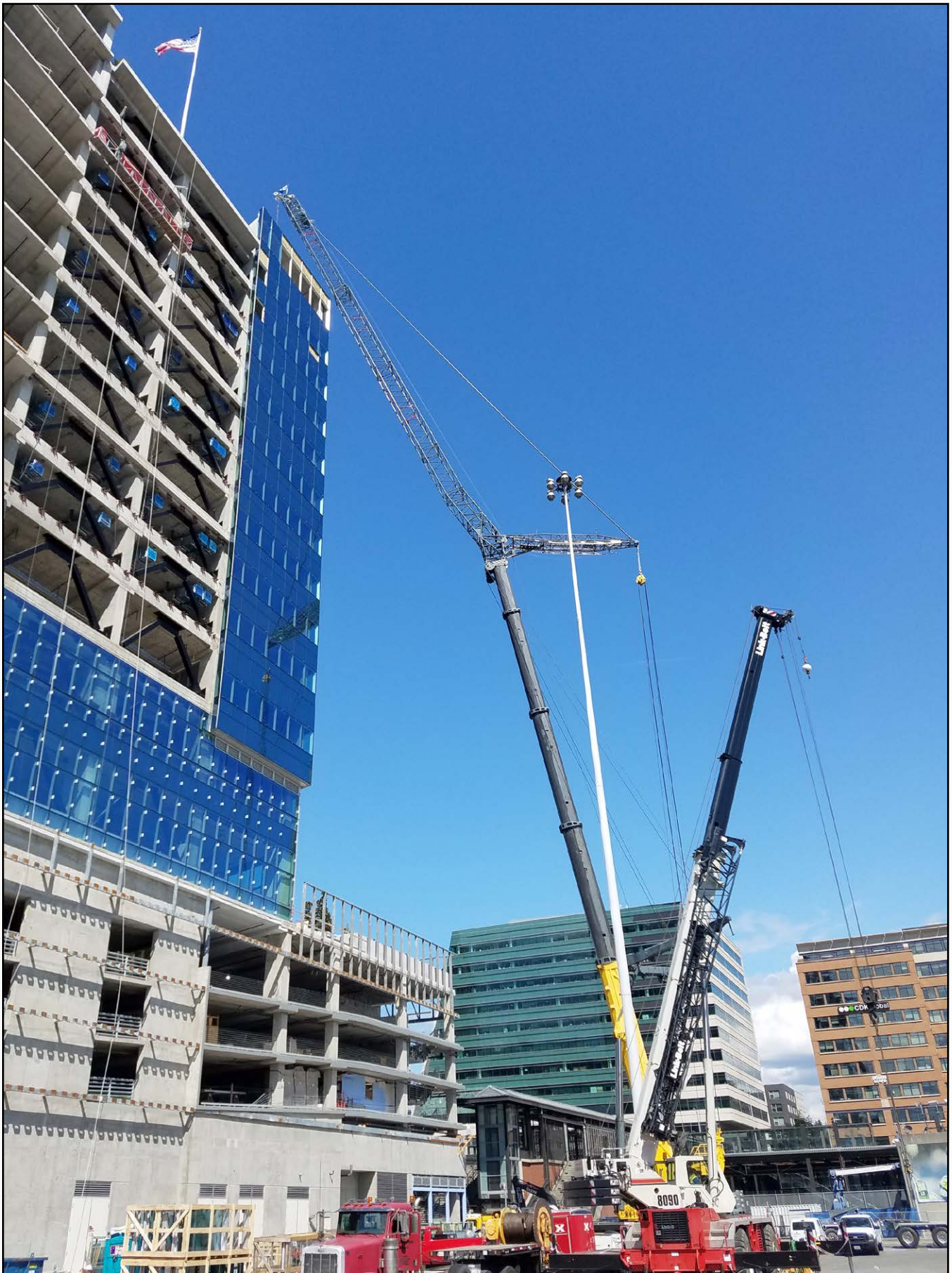
Barnhart's 550 Crew dismantling a tower crane on the 255 S. King St project in Seattle's SODO District
